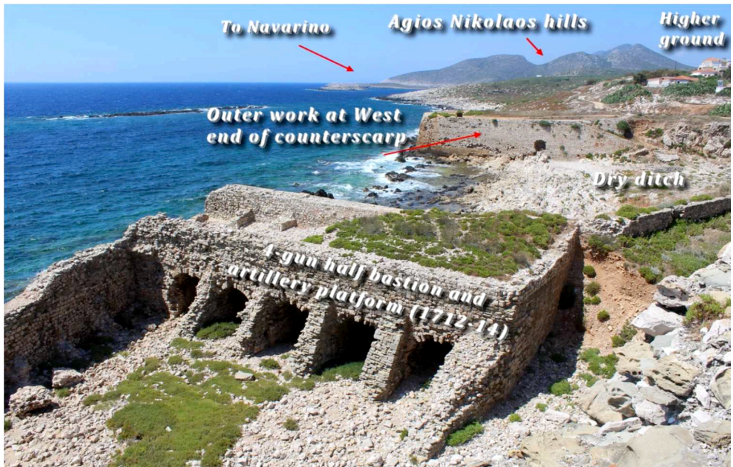
10. New works in the western part of the ditch looking due North, March 2018.
