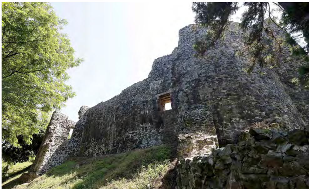
Fig. 2 Giorgi Abdaladze, Ruins of the walls of the Petra Fortress in Tsikhisdziri, Adjara, 17 June 2020, 11:37:33 Communications Department of the Administration of the President of Georgia. CC SA 4.0 International. Wikimedia Commons.
